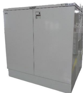
PAD mounted Transformer
