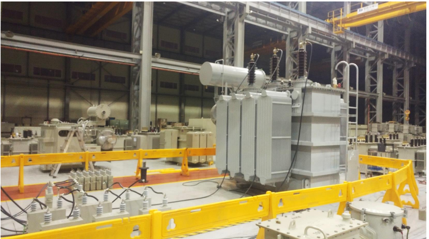
Power transformer testing
